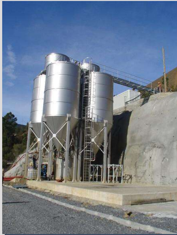
Waste Water treatment facilities
