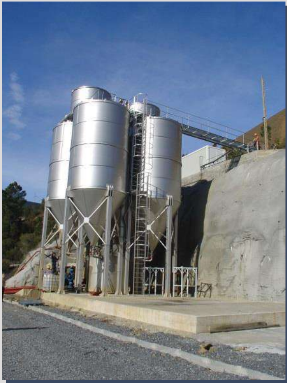
Waste Water treatment facilities
