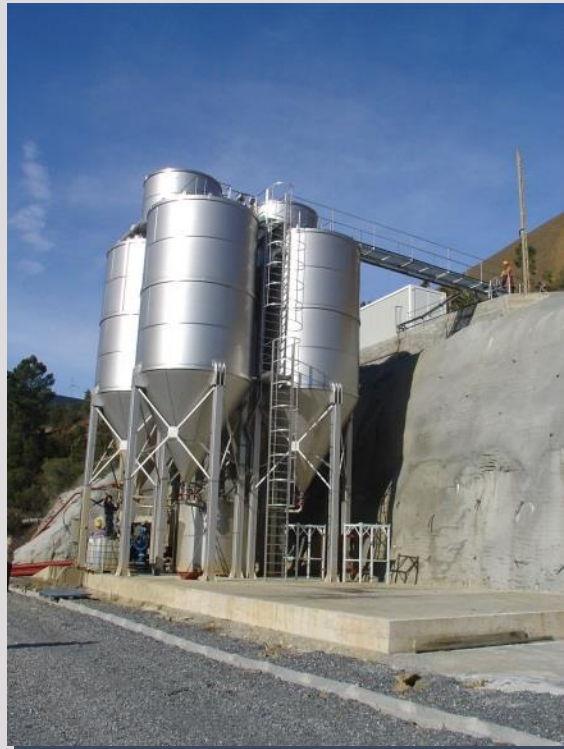
Waste Water treatment facilities
