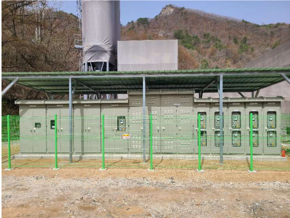
New 4 MW Power System
