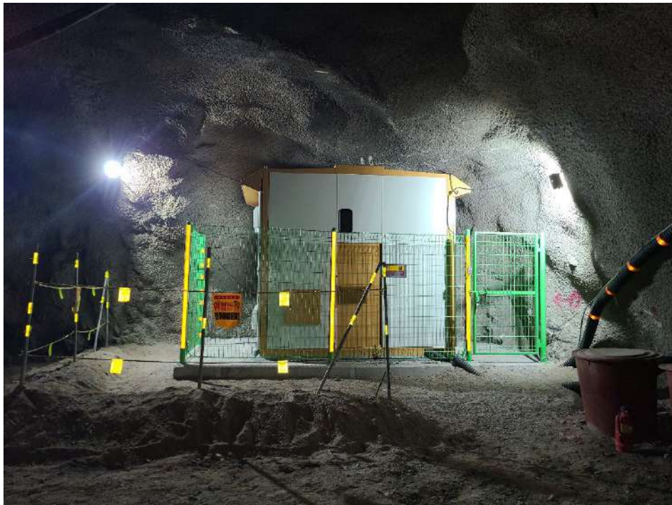
195 KVA Panel Installed Underground at the Sangdong Tungsten Mine
