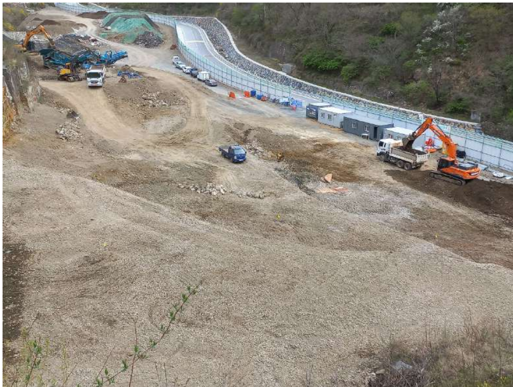
Surface Scalping at the Sangdong Tungsten Mine site, with Temporary Site Offices, New Roads and Drainage in the Background.
