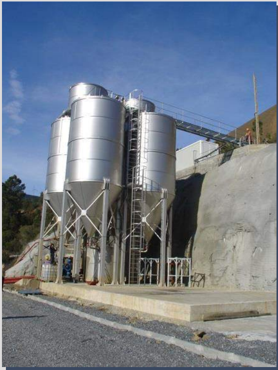
Waste Water treatment facilities
